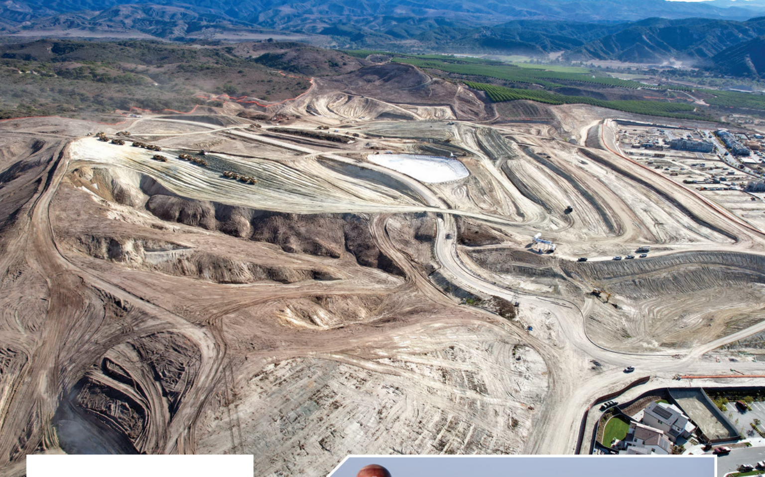
Above: Overview photo of Phase 3 and 4 of the Rancho Mission Viejo Rough Grading and Storm Drain Improvements Project in San Juan Capistrano.
