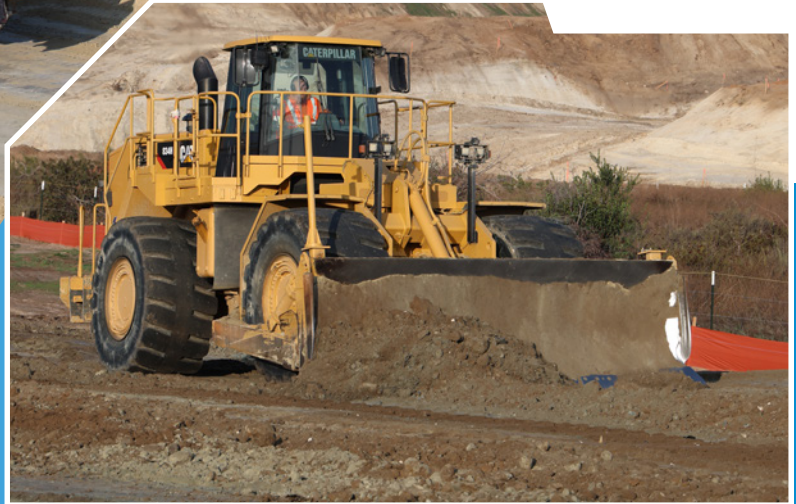
Above Right: LB3 Enterprise's Cat 834 compactor operated by Robert Scudero mixing and compacting the fill on-site.
