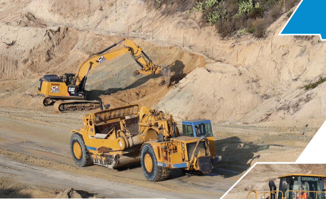
Left: Cat 329 excavator rented from C5 Equipment Rentals excavates a hillside while LB3 Enterprise's Cat 657 scraper returns to the cut on the haul road at the Rancho Mission Viejo jobsite.
