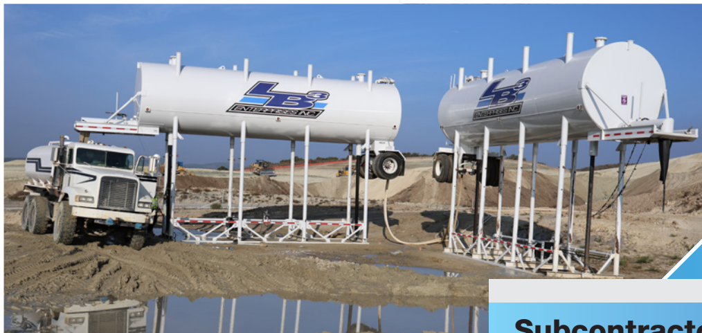
Left: LB3 Enterprise water towers filling one of (subcontractor) Mastiff Equipment Inc.'s water trucks.
